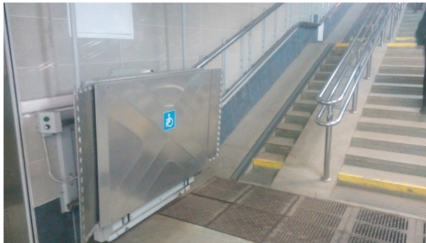
Fig. 1. The lifting platform assisting wheelchair users in one of the pedestrian subways in Minsk, Belarus. (The photograph is the personal property of the article authors.)
